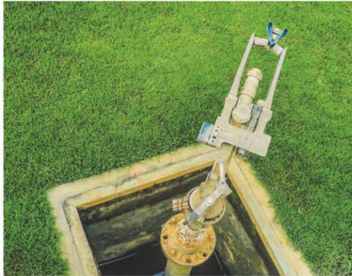
Water Sprinkle System
